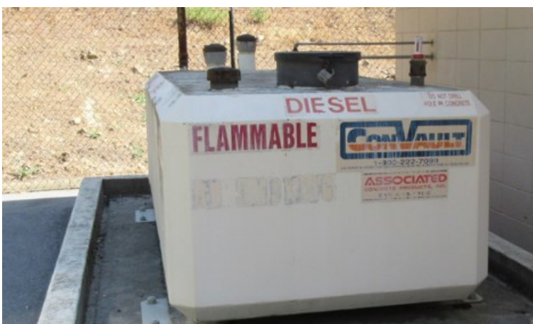
Tank with proper emergency vents and secondary containment
