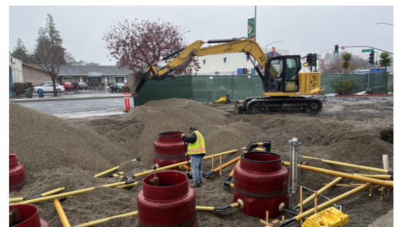
Backfilling a UST with gravel during the installation of a UST system
